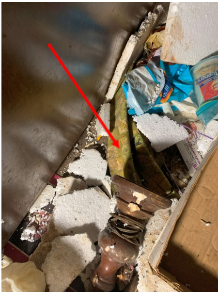
Asbestos-Containing HM# 6 – Floor Sheetting (Cream/Green Pattern)
