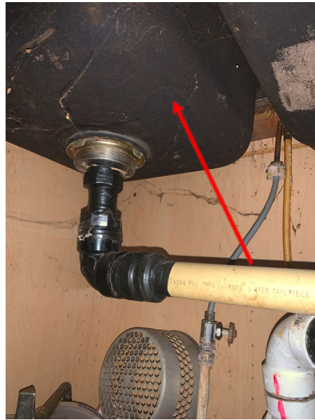
Asbestos-Containing HM# 5 – Sink Undercoat (Black)
