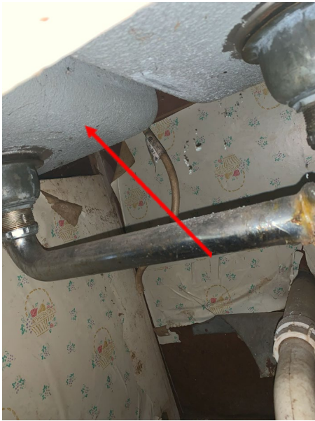
Asbestos-Containing HM# 15 - Sink Undercoat (Grey)
