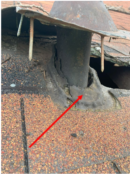
Asbestos-Containing HM #30 - Roof Flashing (Black)
