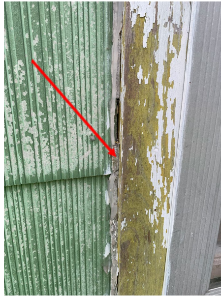
Asbestos-Containing HM #28 - Exterior Caulk (Grey)
