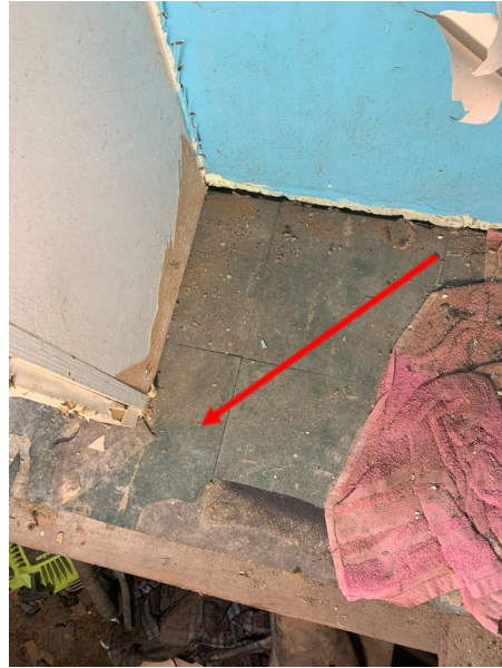
Asbestos-Containing HM# 12 - Multilayer Flooring (Top – White) w/ Tar Paper & Floor Tile (Green) w/ Mastic
