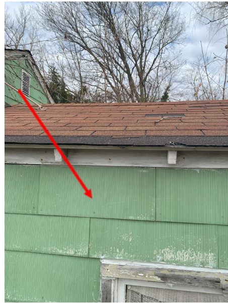
Asbestos-Containing HM #22 - Cementitious Siding (Painted – Green)
