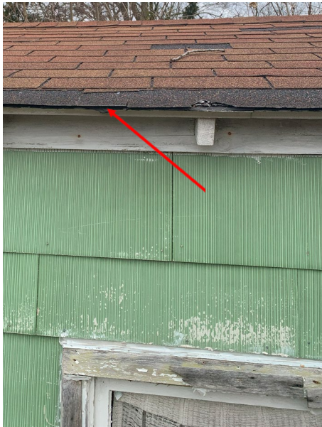
Asbestos-Containing HM #27 - Roof Tar (Black)
